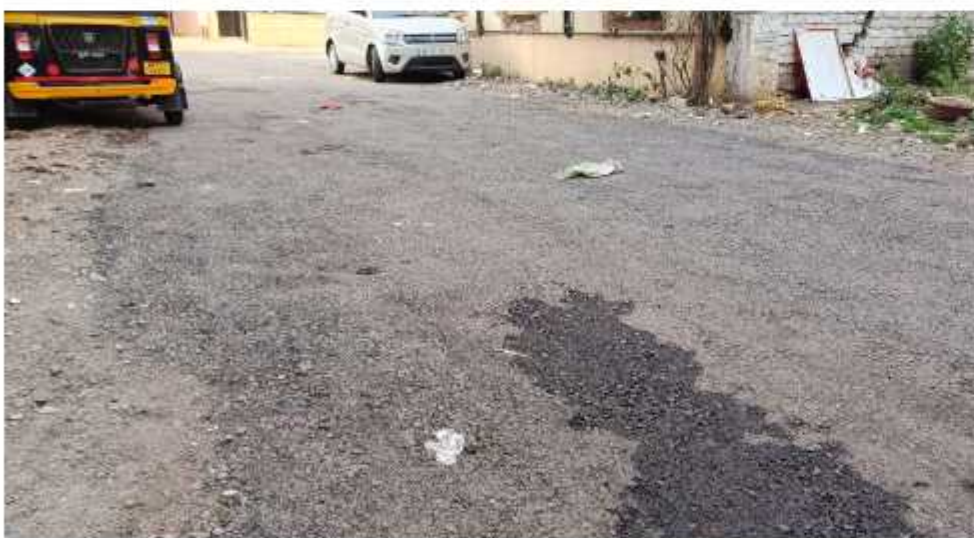
Part of the Sakore Nagar road which was repaired and dug up again.
